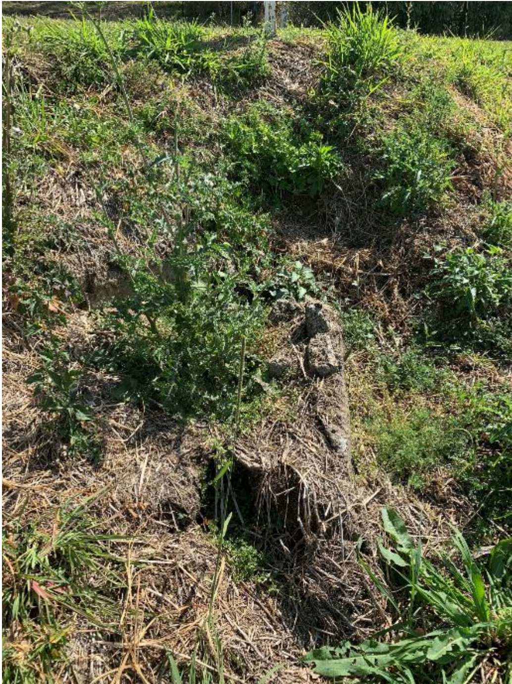
Culvert outlet flowing but obstructed by concrete debris.
