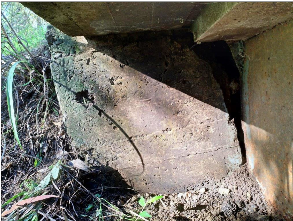
Figure 5: Northern abutment curtain wall cracking and rotation (upstream side)
