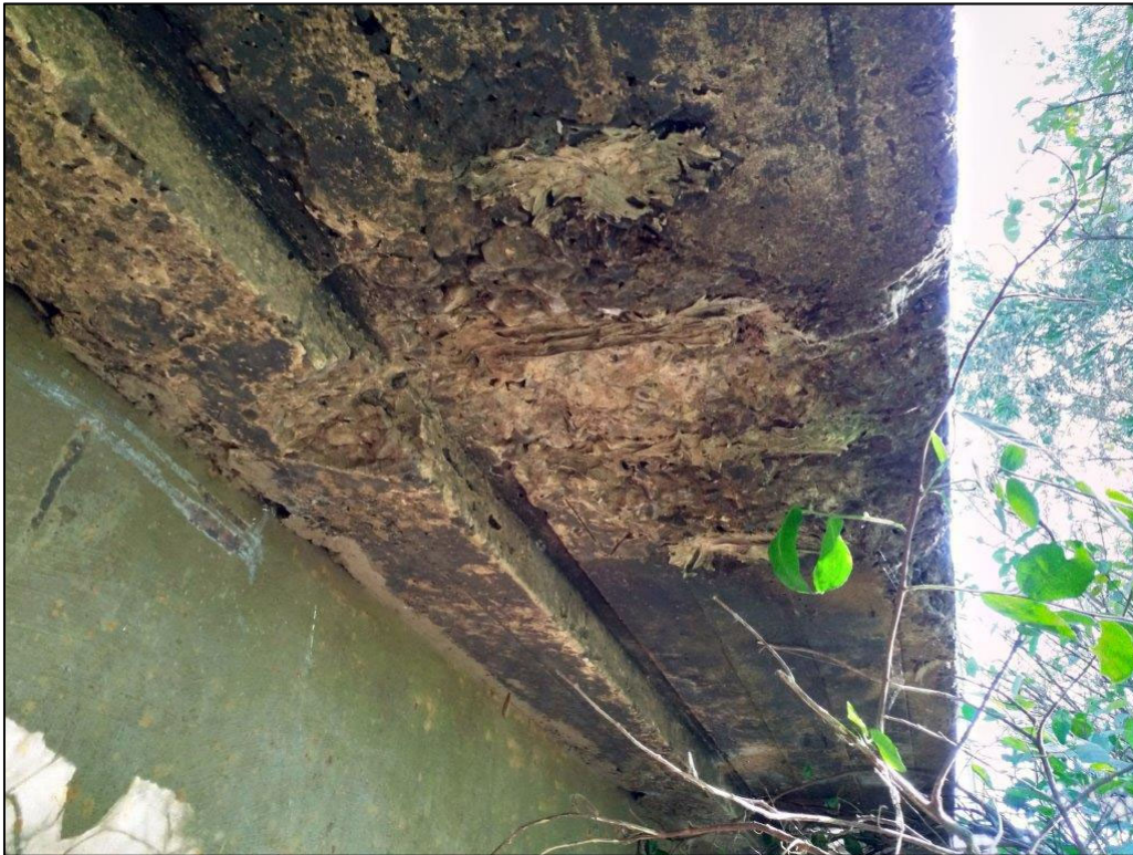
Figure 2: Spalling on underside of deck (upstream, middle)
