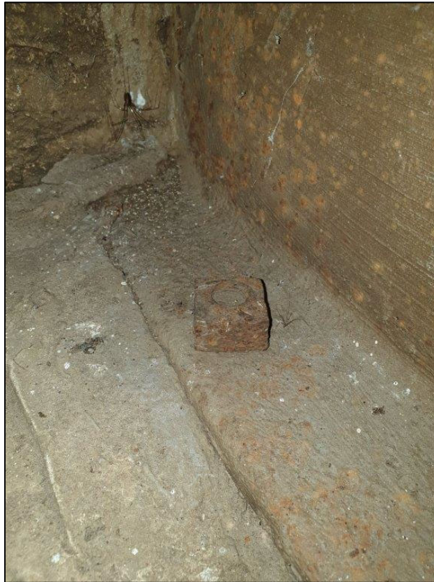
Figure 6: Typical corroded hold down bolt with inadequate thread protruding from nut
