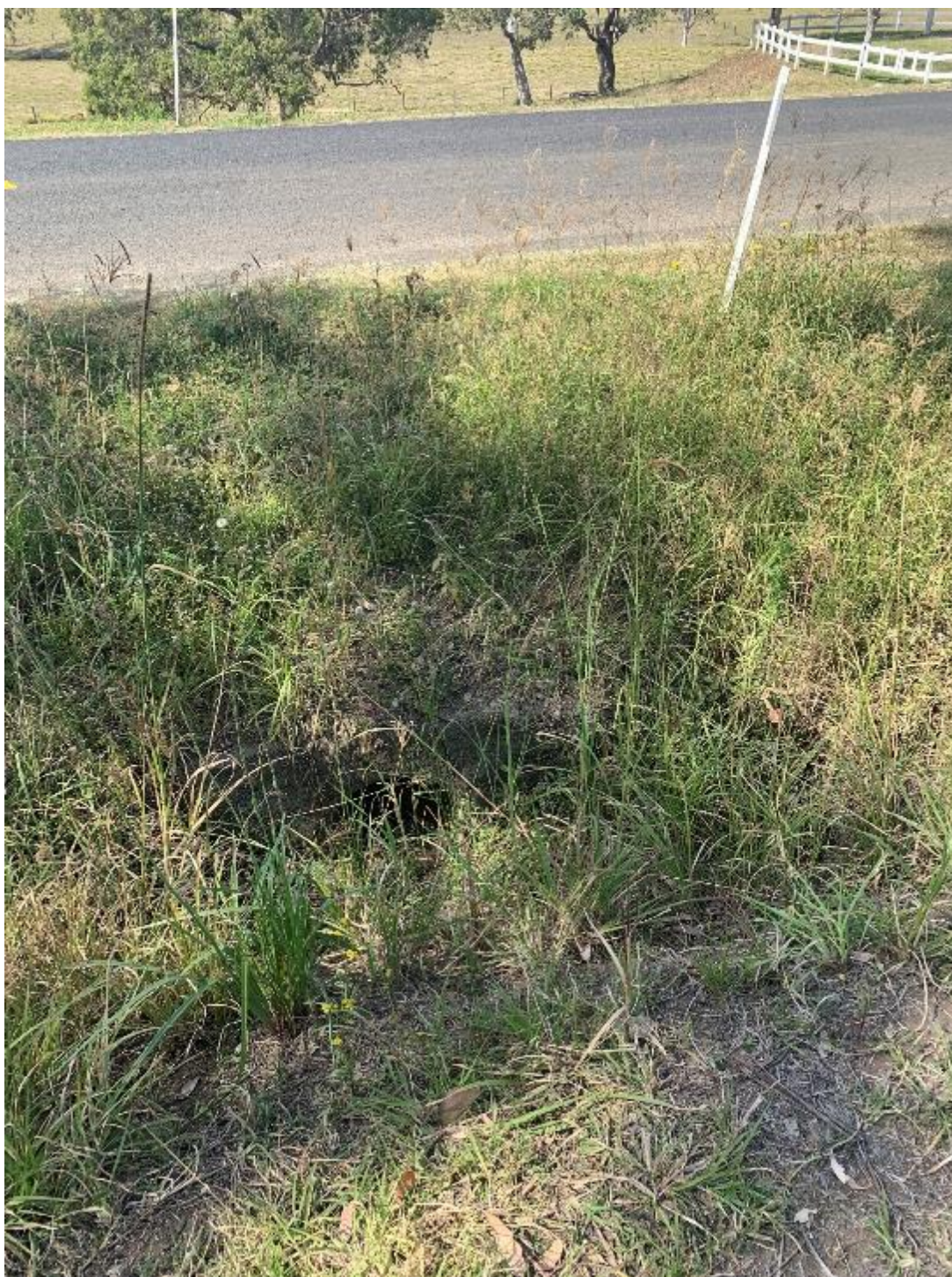
Culvert inlet 50% blocked.
